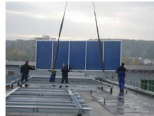
Solar power plant
